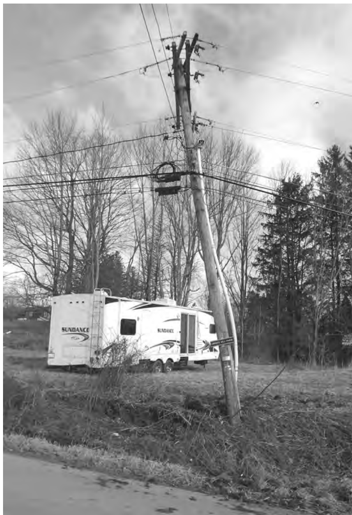
MOVED. This utility pole on Rose Hill Road in Lake Como, PA., apparently bore the brunt of an errant driver over the weekend. It is listing to one side and deep tire tracks and skid marks in the road point to someone going wide of the mark. Herald Photo by Sally Zegers
