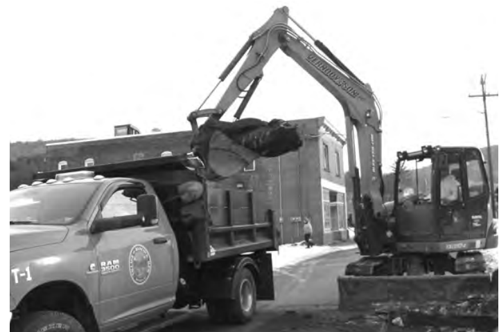
Vernooy & Son backhoe removed the pavement over the suspected water main break on Main Street on December 26.
